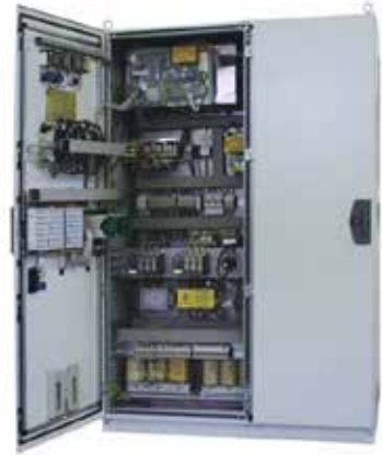
UPS 20 kVA - internal view
